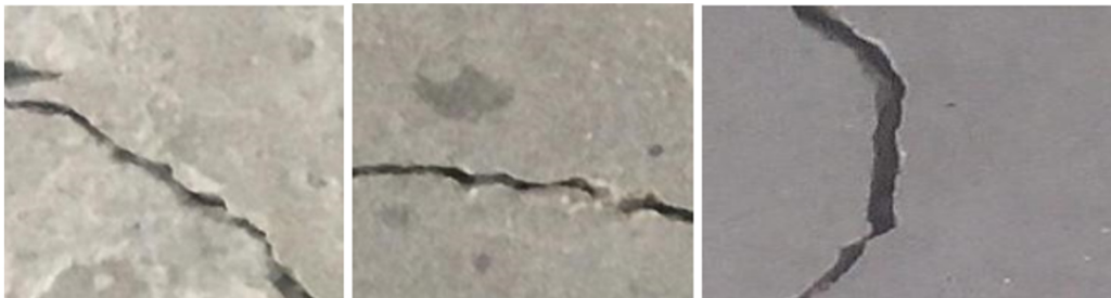
Fig. (1). Surface images with crack.
