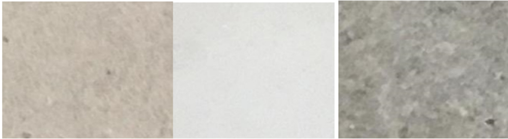
Fig. (2). Surface images without crack.
